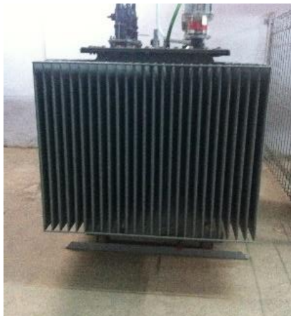
Gambar 1. Transformator 20/0.4 KV, 50 Hz, 800 KVA oil immersed,
